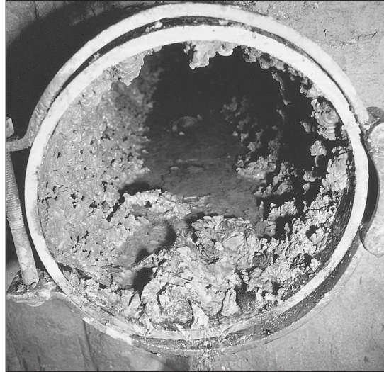
Figure 1-1 Pipe with tuberculation caused by corrosion
