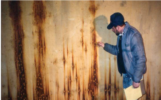
FIGURE 1-3 Vertical Corrosion of Interior Tank Wall
