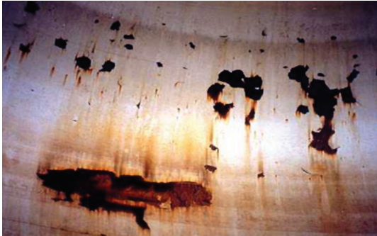
FIGURE 1-4 Corrosion at Coating Holidays
