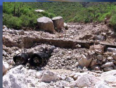
Massive damage to the road and culverts near Tram Stop #8 in Sabino Canyon. (Photo by Chris Magill, USGS, 8/8/06)
