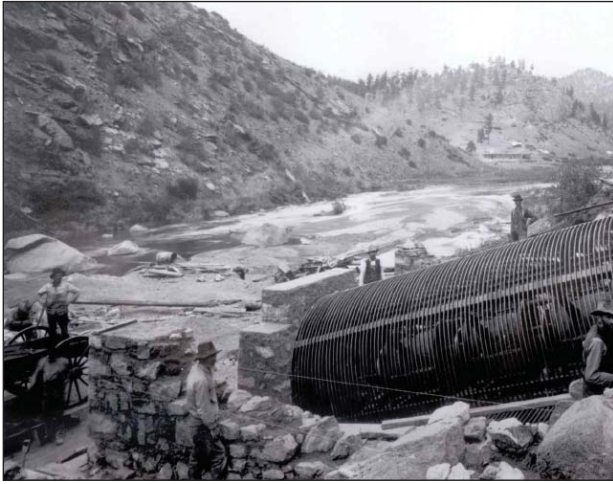
Denver Water engineers used old blueprints and original construction photos to compile construction documents that would accurately reflect the work underwater divers needed to do to rehabilitate the 105-year-old Cheesman Dam, located about 50 miles southwest of Denver.
