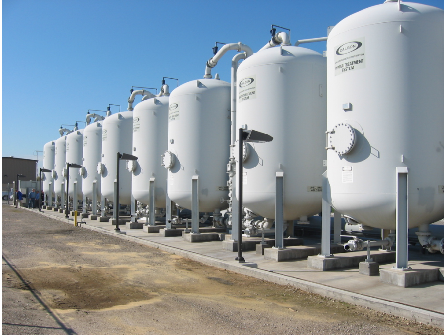
Figure 3-5. Single Pass Ion Exchange System Installed at California Domestic Water Co.
